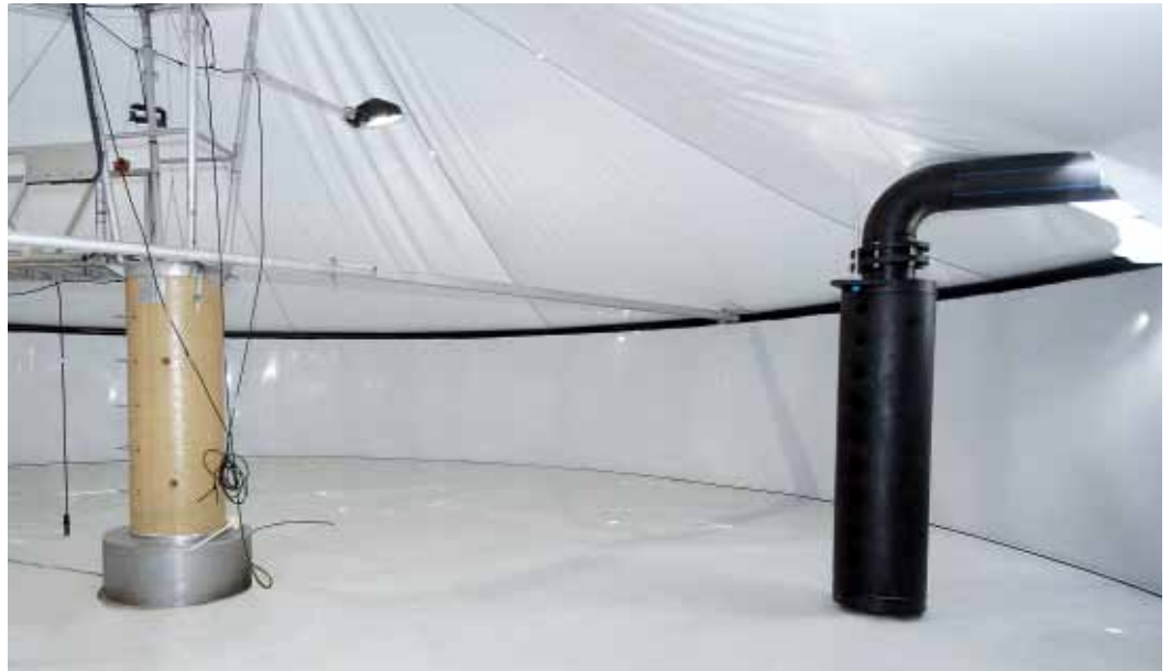
SOLVOX ® OxyStream in a 15-m-diameter tank at Marine Harvest's site in Glomfjord, Norway.
