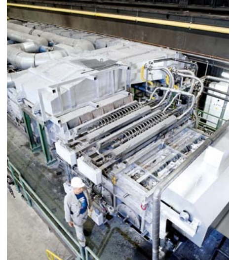
Three metres of the recuperative zone was used to fit the compact DFI oxyfuel unit.
