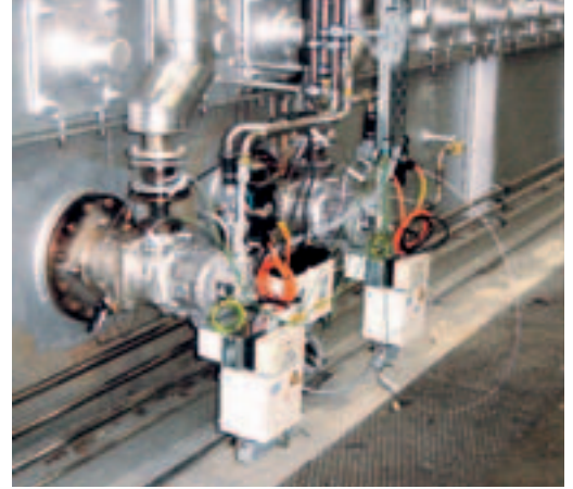
Installation of CARBOCAT® (roller hearth furnace)
