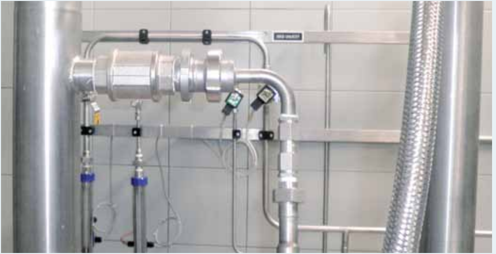
Installation of the SOLVOCARB® inline injector at the Plzeňský Prazdroj brewery.
