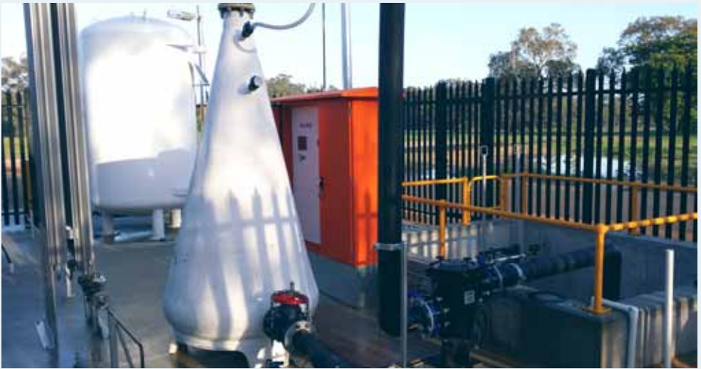
SOLVOX C-110 installation at one of the four oxygenation plants on the Canning and Swan rivers.
