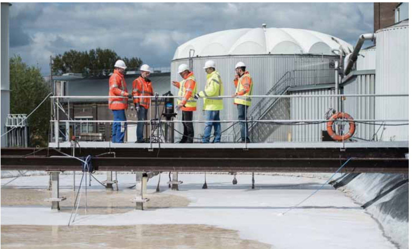
SOLVOX mobile installation at an industrial wastewater plant in the Netherlands.
