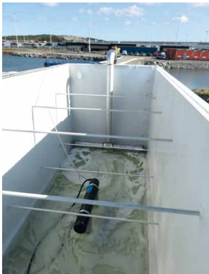
SOLVOCARB® mobile installed in the neutralization tank during commissioning
