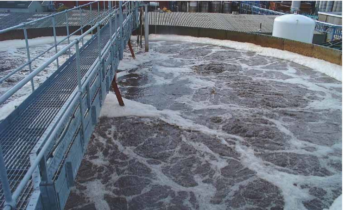
Pure oxygen creates optimal aerobic conditions for successful biological treatment and faster degradation rates, and it supports biological nutrient removal.
