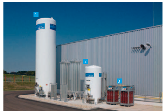
Gas supply station including nitrogen tank, argon tank and acetylene cylinder packs.
