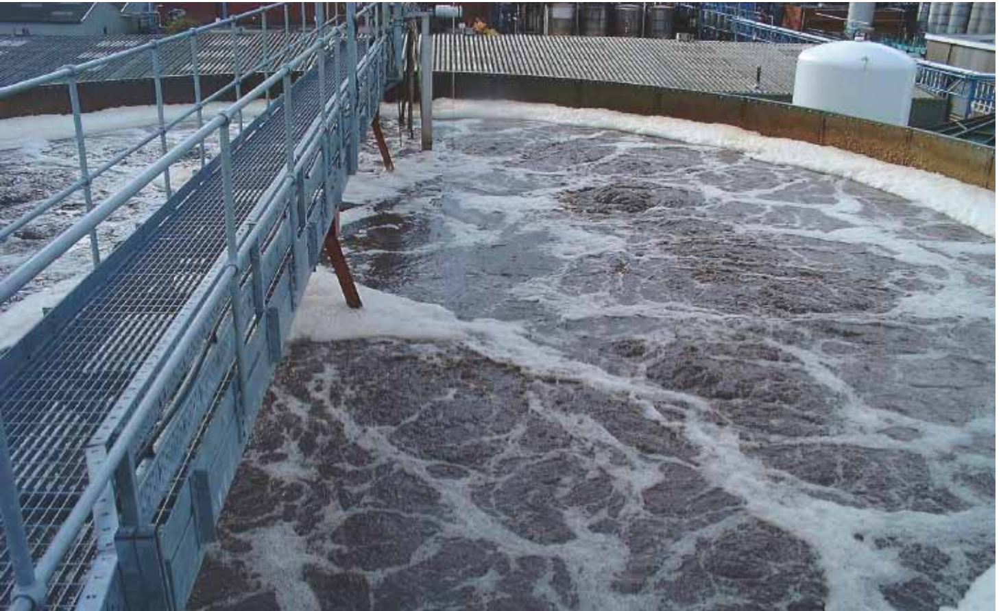
Pure oxygen creates optimal aerobic conditions for successful biological treatment and faster degradation rates, and it supports biological nutrient removal.
